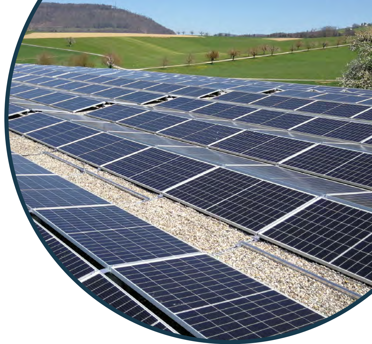
Solar plant in Brislach (Switzerland)
